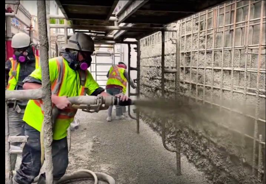
Shotcrete is very hazardous and wasteful.
